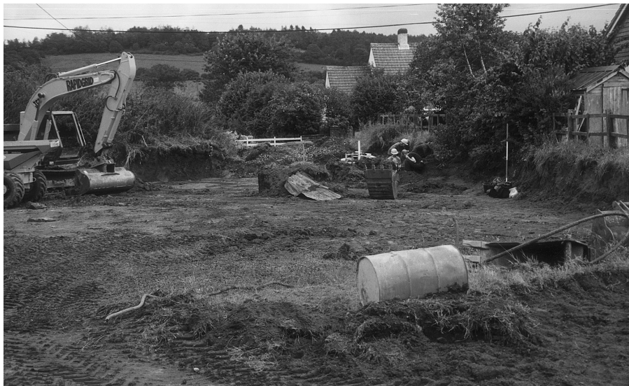
Plate 1: Site 2, plot 118. Rescue work on the site of a 13th/14th-century house, destroyed before the planning authority intervened, looking towards the Catbrook road. The well containing 14th-century remains was left intact. Copyright: Monmouth Archaeology.
