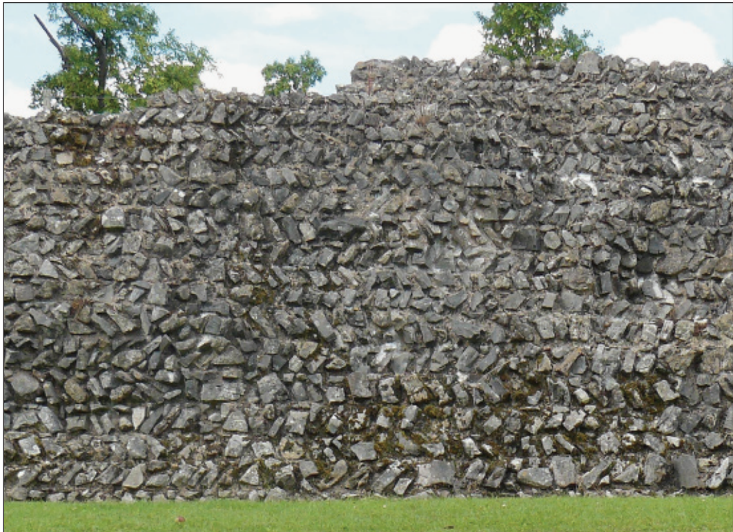
Fig. 13. Herringbone work in South-east Wall at Caerwent, c. 60m from northern end of section. The wall survives here to a height of c. 3.5m.
