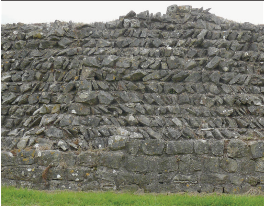
Fig. 2. Portion of South-west wall of Caerwent, c. 45m south of West Gate, to show residual outer facing, core and a large marker at a divergence. The wall survives here to a height of c. 2.5m. See also Fig. 9.
