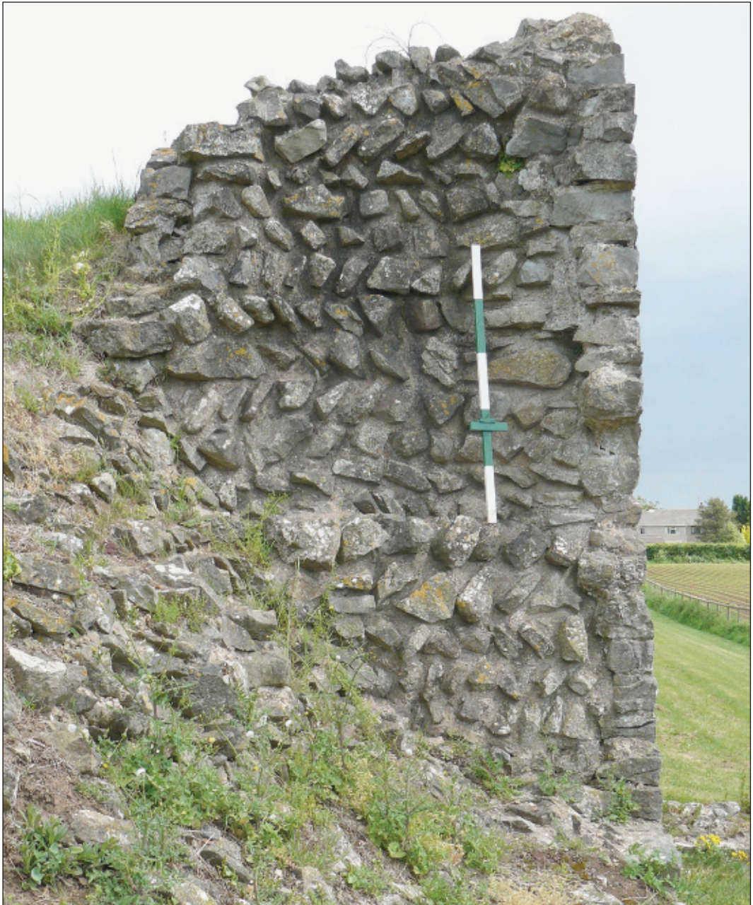
Fig. 8. Cross-section of the wall at No. 5 Bastion exhibiting shingled courses aligned transversely to the line of the wall. See also Fig. 11. Scale 1.25m.
