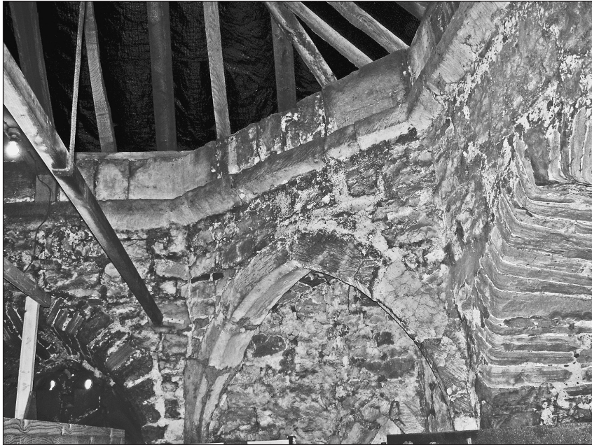
Fig. 10. The north-west belfry squinches of the tower of Caldicot parish church in 2008, looking west.
