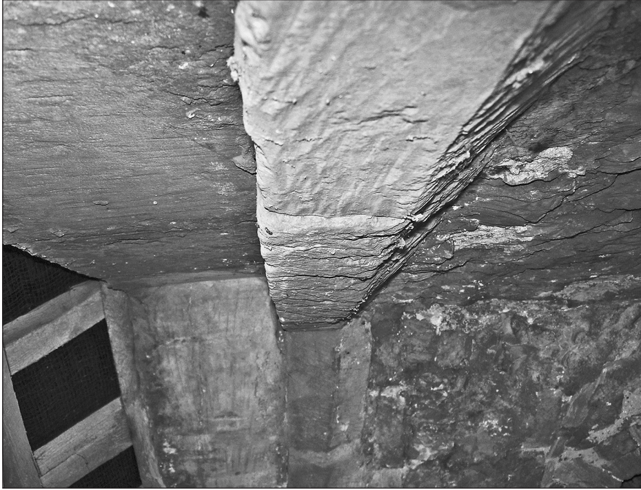
Fig. 13. The south-eastern corner of the belfry of the tower of Caldicot parish church looking east, in 2008, showing the first course of the intended spire.
