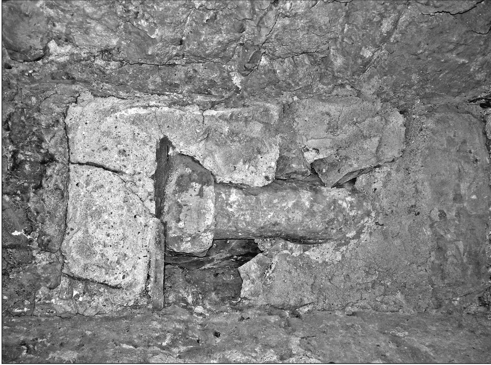
Fig. 7. The western, blocked, slit of the third storey of the tower of Caldicot parish church in 2008.
