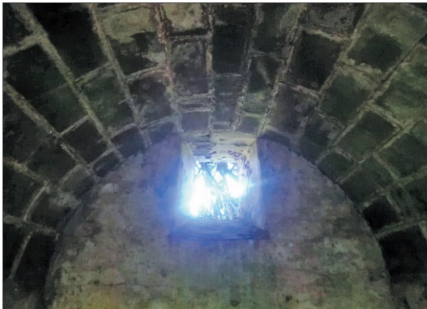
Fig. 5: The north wall's window close to the barrel roof of Cadw's 'game larder'. © Ann Benson
