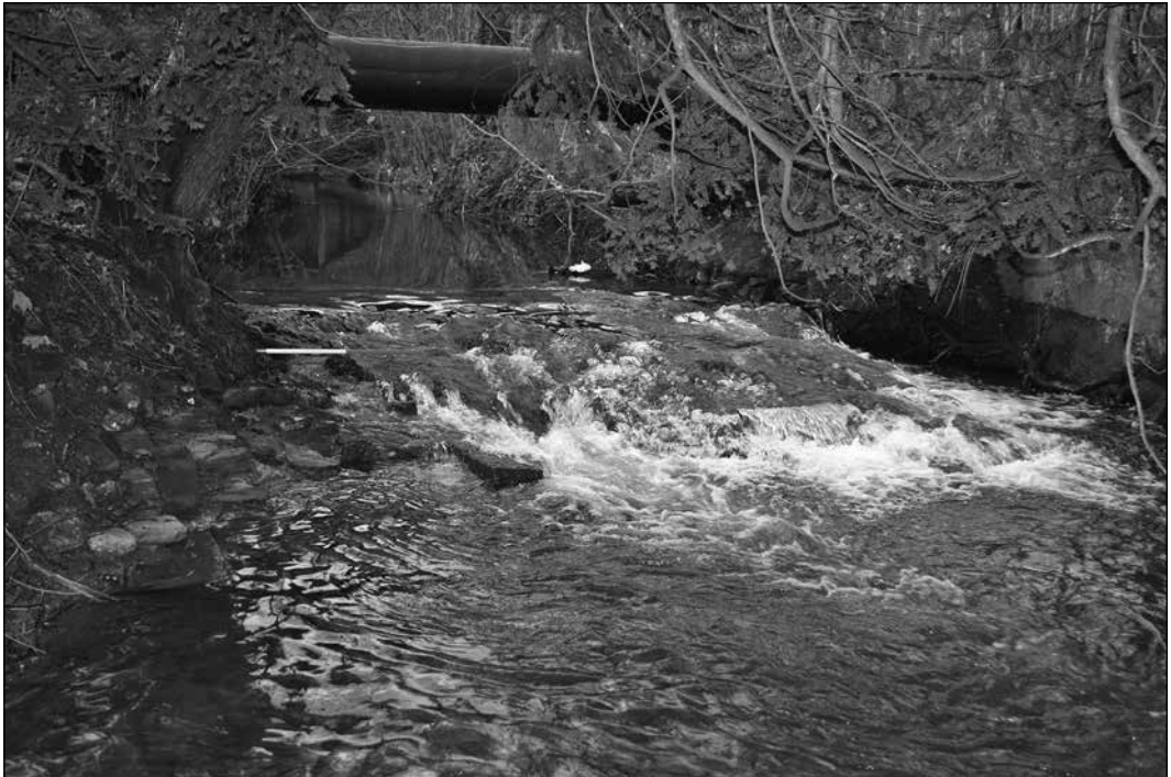
Plate 3: Looking upstream from the southern bank at site 9. Measuring just over 6m wide and holding evidence for up to three sluice gates, this bridge would have been a vital communication and supply route during the medieval period. Photograph: D. Standing.
