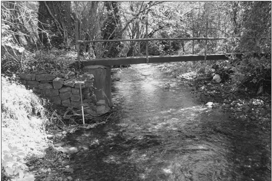
Plate 1: Site 3a was at least 2m wide while extending 1.5m into the current bank. Photograph: D. Standing.
