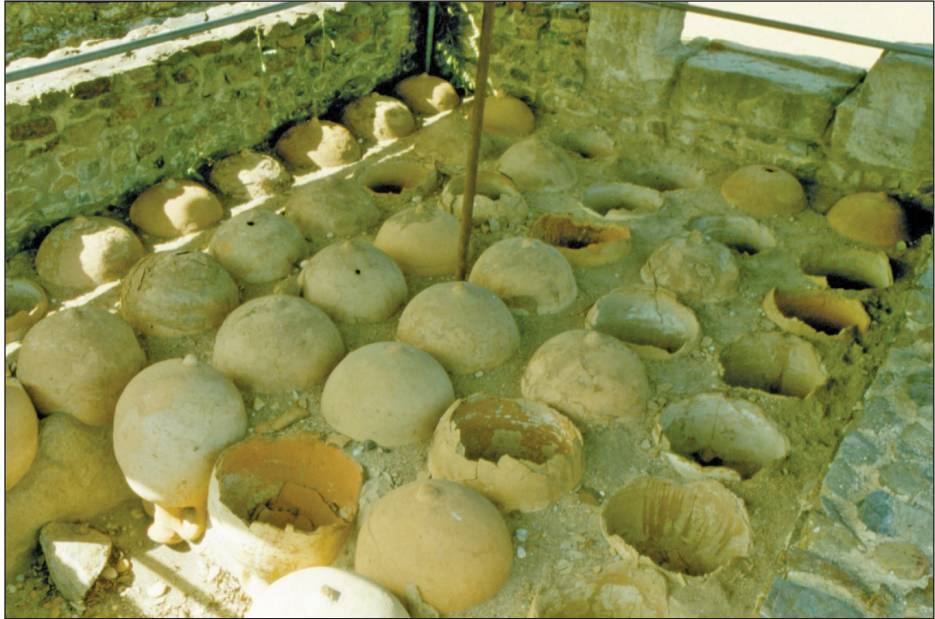
Fig. 8: Globular oil amphorae used as a damp course in a shop building at St. Romain-en-Gal. Photographed by the author.
