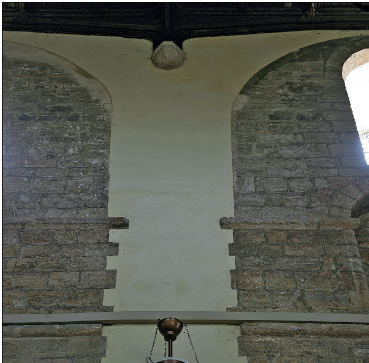
Fig. 6. Chepstow Priory, S nave, detail of clerestory string and arcs of former high vault above pier S3.
